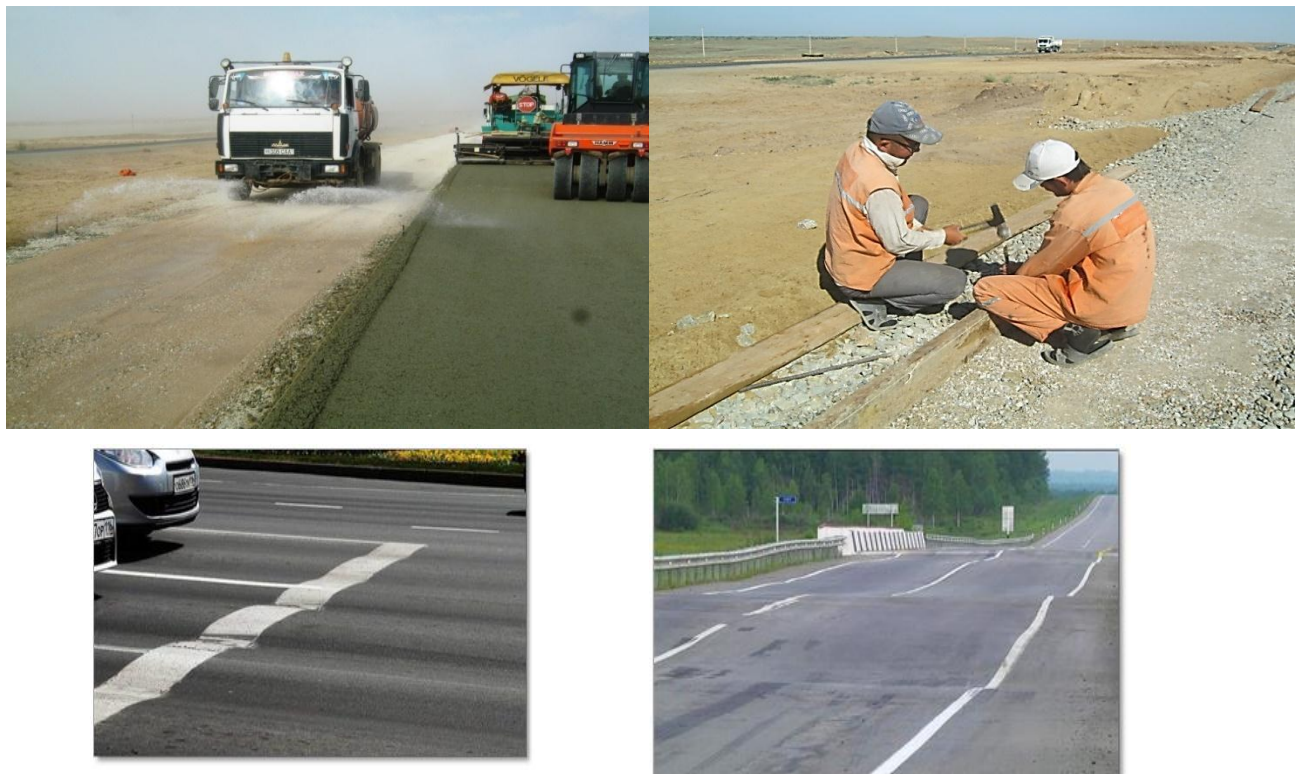
The process of applying the base and additional layers and coatings (photo by the author)
